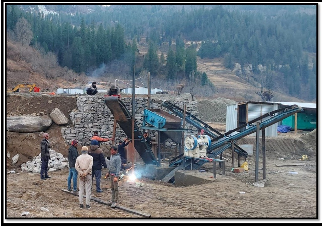
Figure 18: Crusher Plant installed at head works
